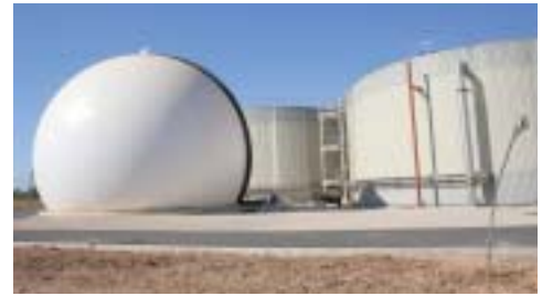
submersible stirrer for homogenizing the mixed sludge.
